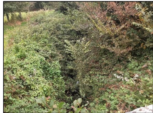
Plate 6- 40 Overgrown channel of Ballyhennessy_23 of watercourse
