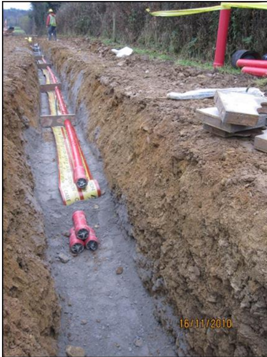
Plate 4.12 Cable Trench and Conduit
