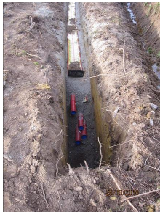
Plate 4.13 Cable Trench and Conduit
